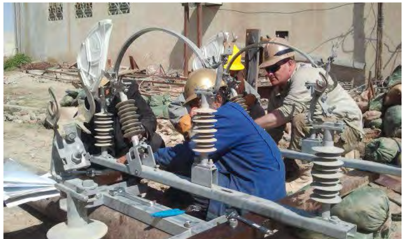
A U.S. Army Corps of Engineers official and an Afghan utility technician assemble the air disconnect at the Sangin substation.
